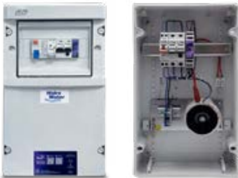
Space saving in the electrical box
