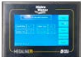
Large format control panel
