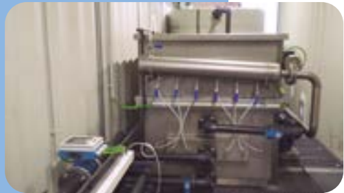
DAF in container
